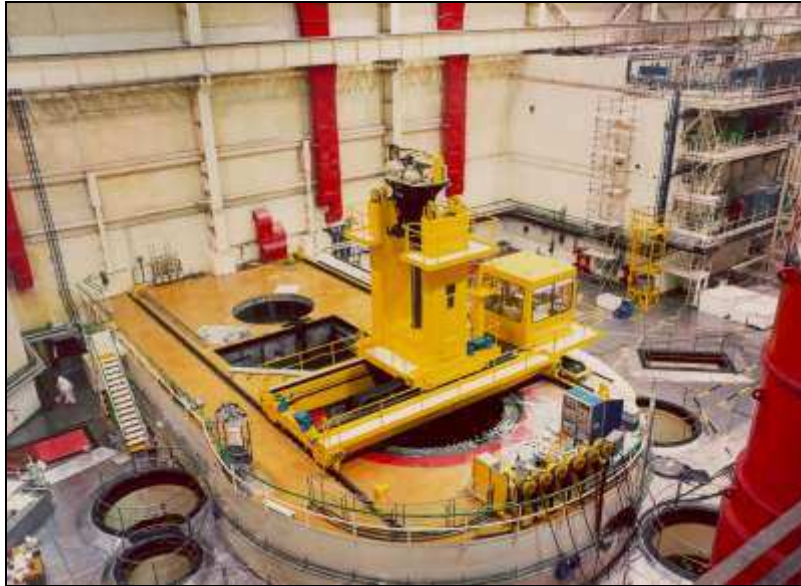
Fig. 4.1 Uncovered SF pool and ŠTK during reactor refueling
