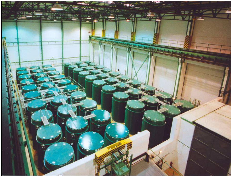
Fig. 4.2 Fully occupied storage hall in ISFSF Dukovany
