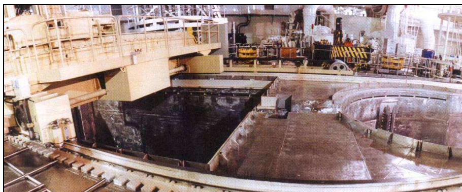
Fig. 4.3 Uncovered SF pool at NPP Temelín
